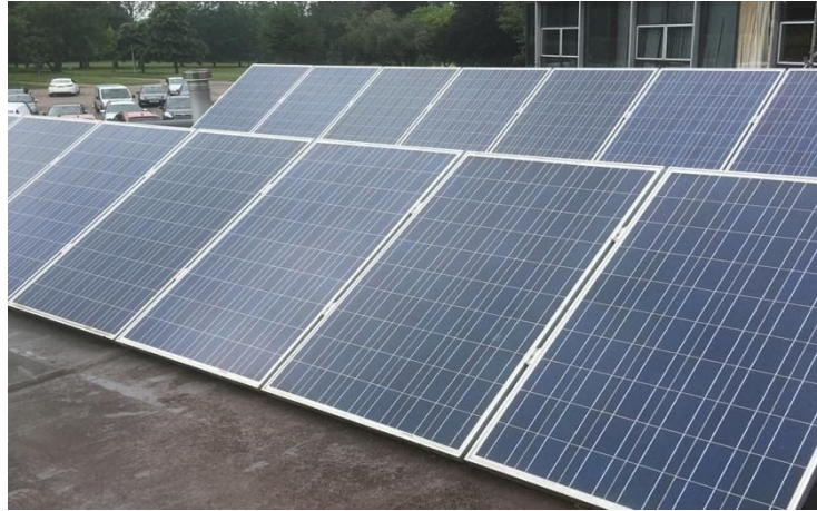
Photovoltaic Panels Clubhouse Roof
